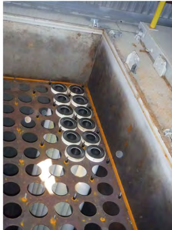
Ceramic filters with venturi installed
